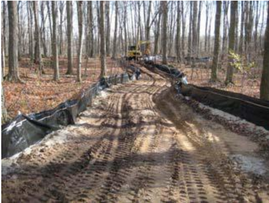
Photo 13 – View showing the buried feeder line to Recharge Well RW317D, after backfilling. Extra feeder lines are typically buried at the same time; if additional recharge wells are subsequently required then less trenching will be necessary. GHD 2012-11-14
