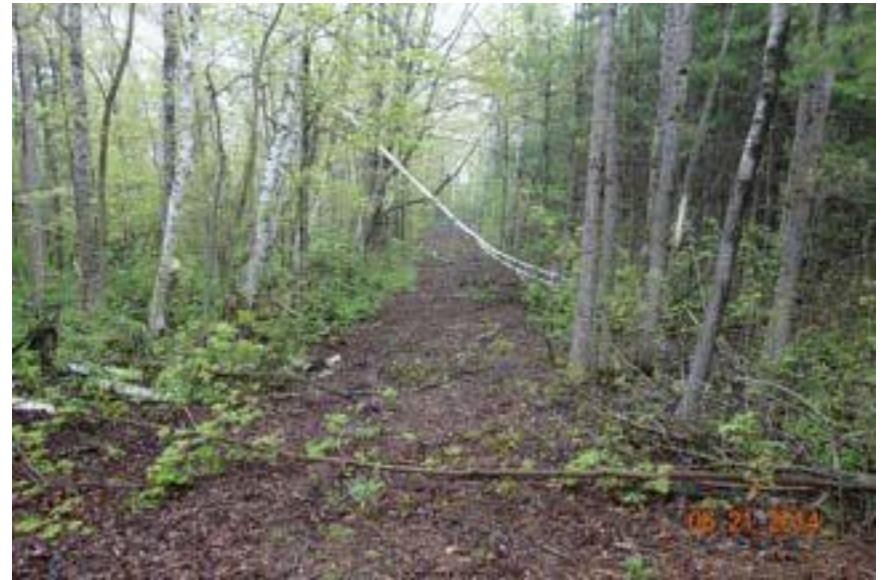
Photo 18 – View of buried feeder line leading to Recharge Well RW206C. This photo was taken 5 years after the feeder line was installed. Note the woody debris and native ground flora along the feeder line alignment. GHD 2014-05-21
