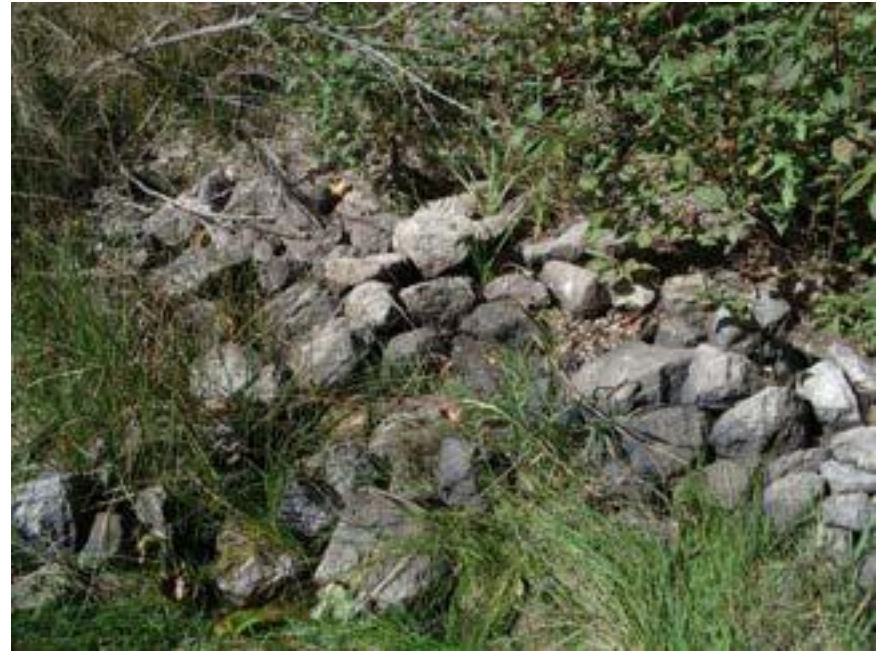
Photo 28 – View showing Wetland W7 Diffuse Discharge Inflow. Note that the gabion stone used to armour the diffuse discharge is now well-weathered, 7 years after it was installed. GEC 2017-10-01
