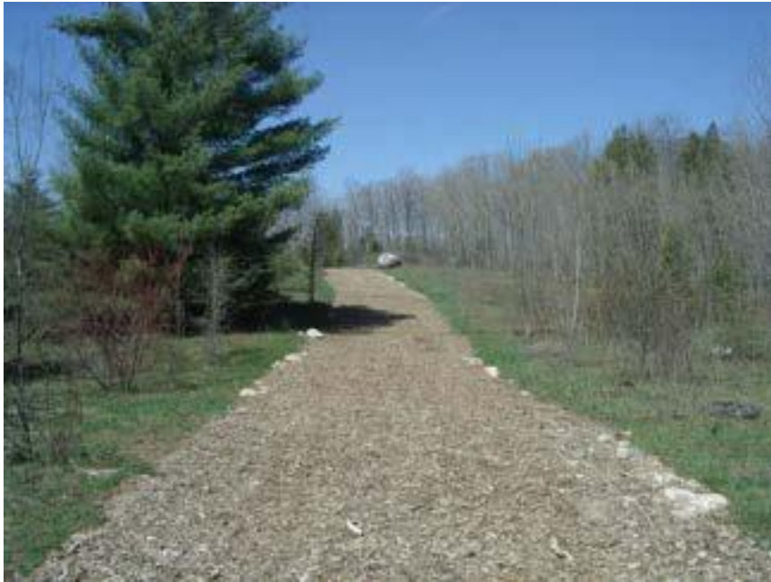
Photo 9 - View showing recently buried feeder lines leading to Recharge Wells RW203C, RW203D, RW204C and RW204D, with a 15-20 cm deep layer of fresh wood chips. GEC - 2013-05-04
